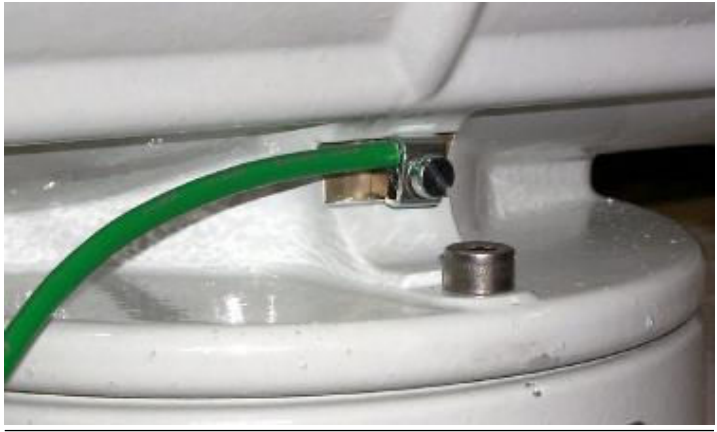
Figure 1-8: Ground Wire Removed
